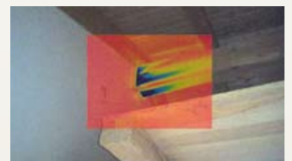
Air leak during blower door inspection, Picture in picture image
