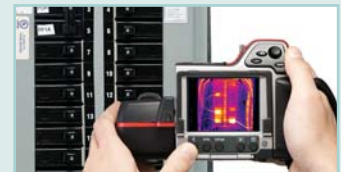
Infrared cameras quickly locate problems with electrical equipment
